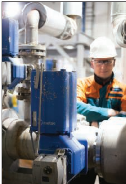
FIGURE 2. Correct control-valve selection enables seamless process operation, even in demanding process or environmental conditions
